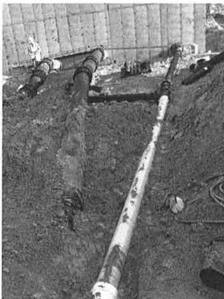
From Left-Outlet, Inlet and Overflow
