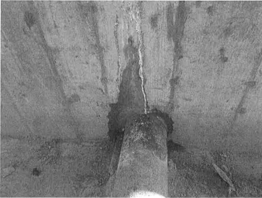
Seep at Outlet Pipe-Morning
