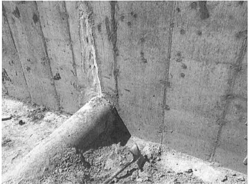
Seep at Outlet Pipe-Afternoon
