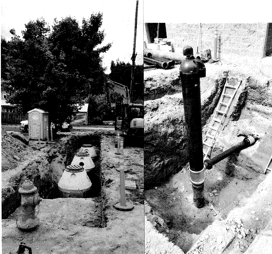
Pump discharge basin west of well house. Well pump connection to well house.
