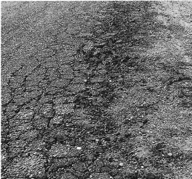
Example of deteriorating condition of pavement.
