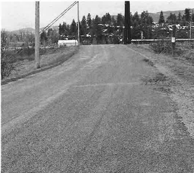
(5) Near the western end of project, facing west. Note the city wastewater bridge.
