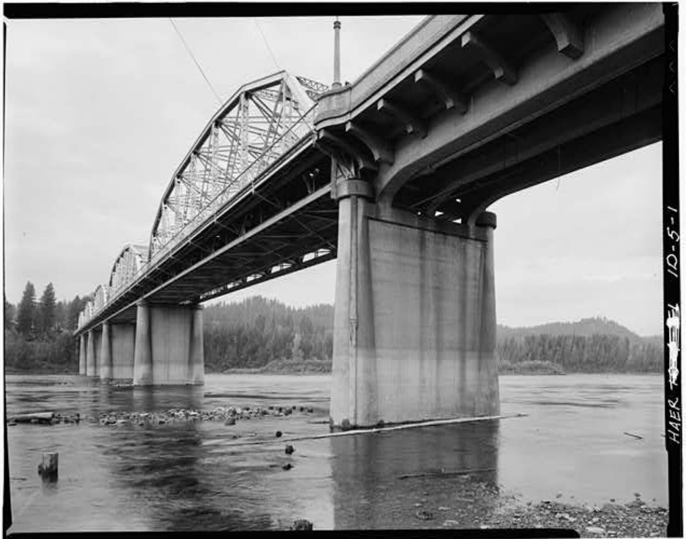
Bonners Ferry Bridge, Spanning Kootenai River, Photo Source: Library of Congress Prints and Photographs Division
